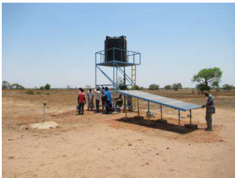
Passy Chally LBS, water supply + solar installation.
