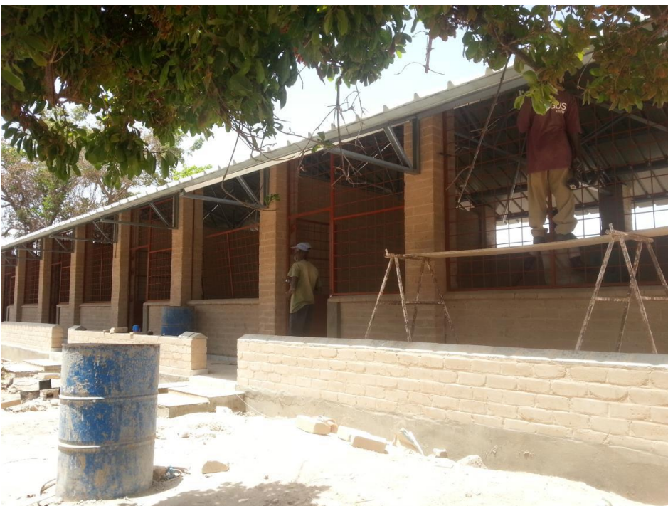
Above: A new nursery school next to the Gambia college (PABO). A project in collaboration with “stichting Bouwen”.
