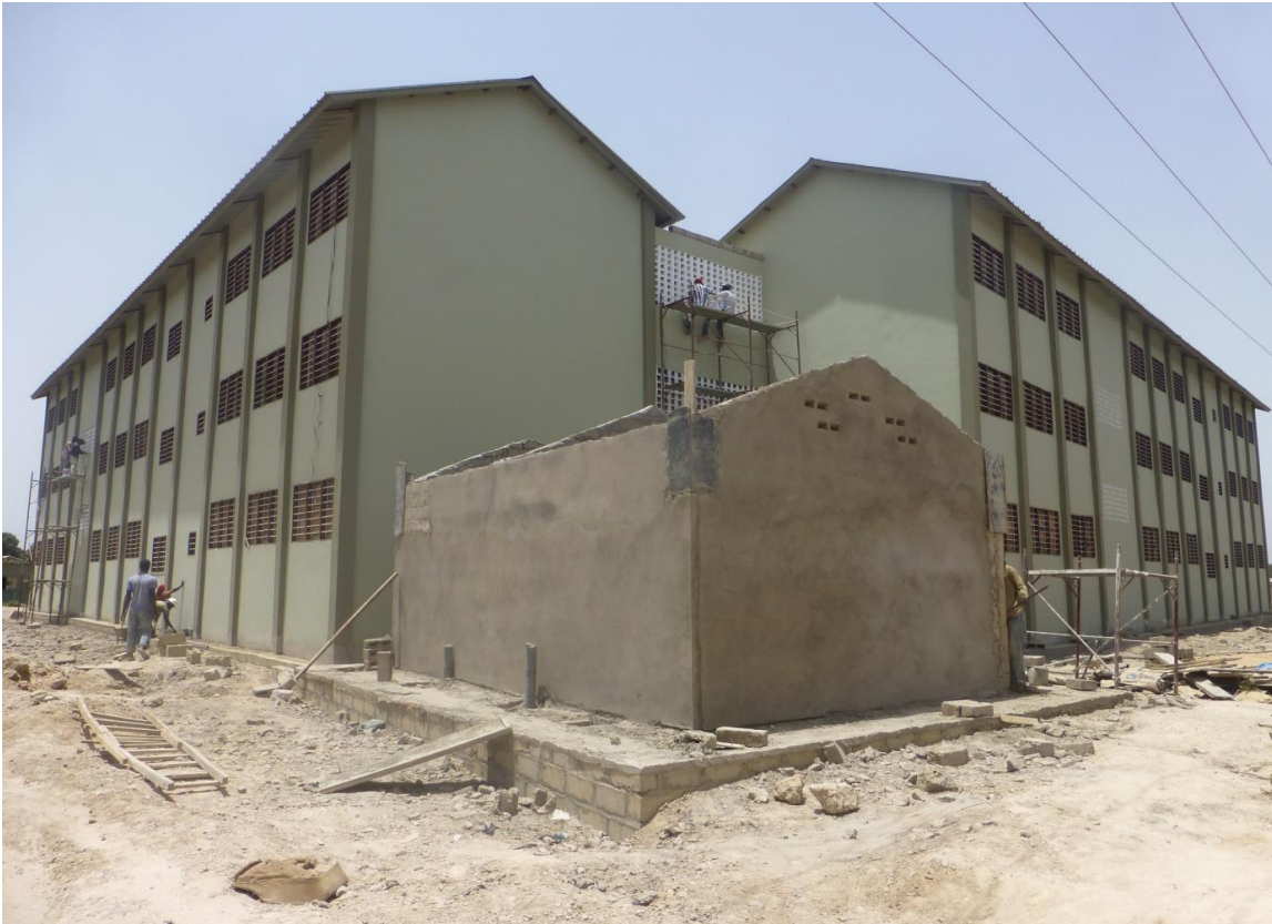
Nema Kunku; First 18 class rooms of this new Lower Basic School are almost finished and will be in use from September onwards. The second phase with another 18 classrooms for a new upper and senior school has started in June.
