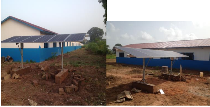
Below: The new building (18 classrooms) for Kabafita Senior Secondary School (opened in November 2018)
