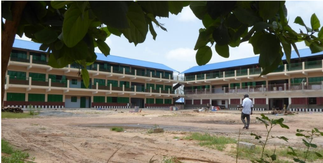
Below: The new building (30 classrooms) in construction for Kabafita Annex Lower Basic School.
