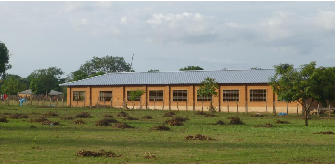
In Tumani Tenda the first three classrooms for the Upper Basic School are ready. Contractor Jan Bos.
