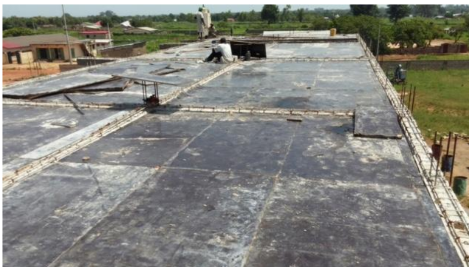
Preparation of the floor for the second level in Kombo Kerawan, contractor Papa Omar Jarju
