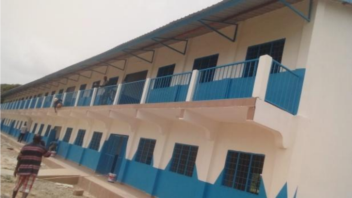
Construction work at Giboro is accomplished and classroom ready to be used.
