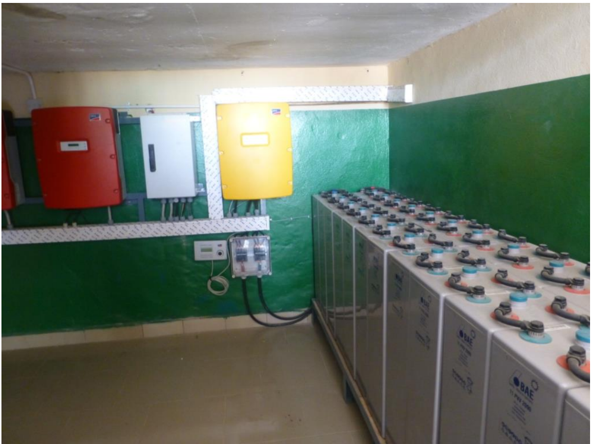
Batteries for the new solar system of the basic school in Sifoe.
