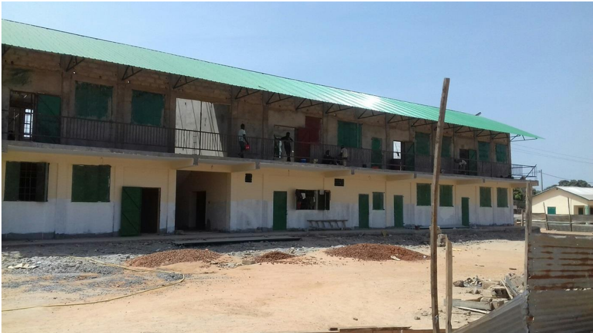
The new school building in Mandinary that will be taken into use in September 2016. Picture 26-05-2016
