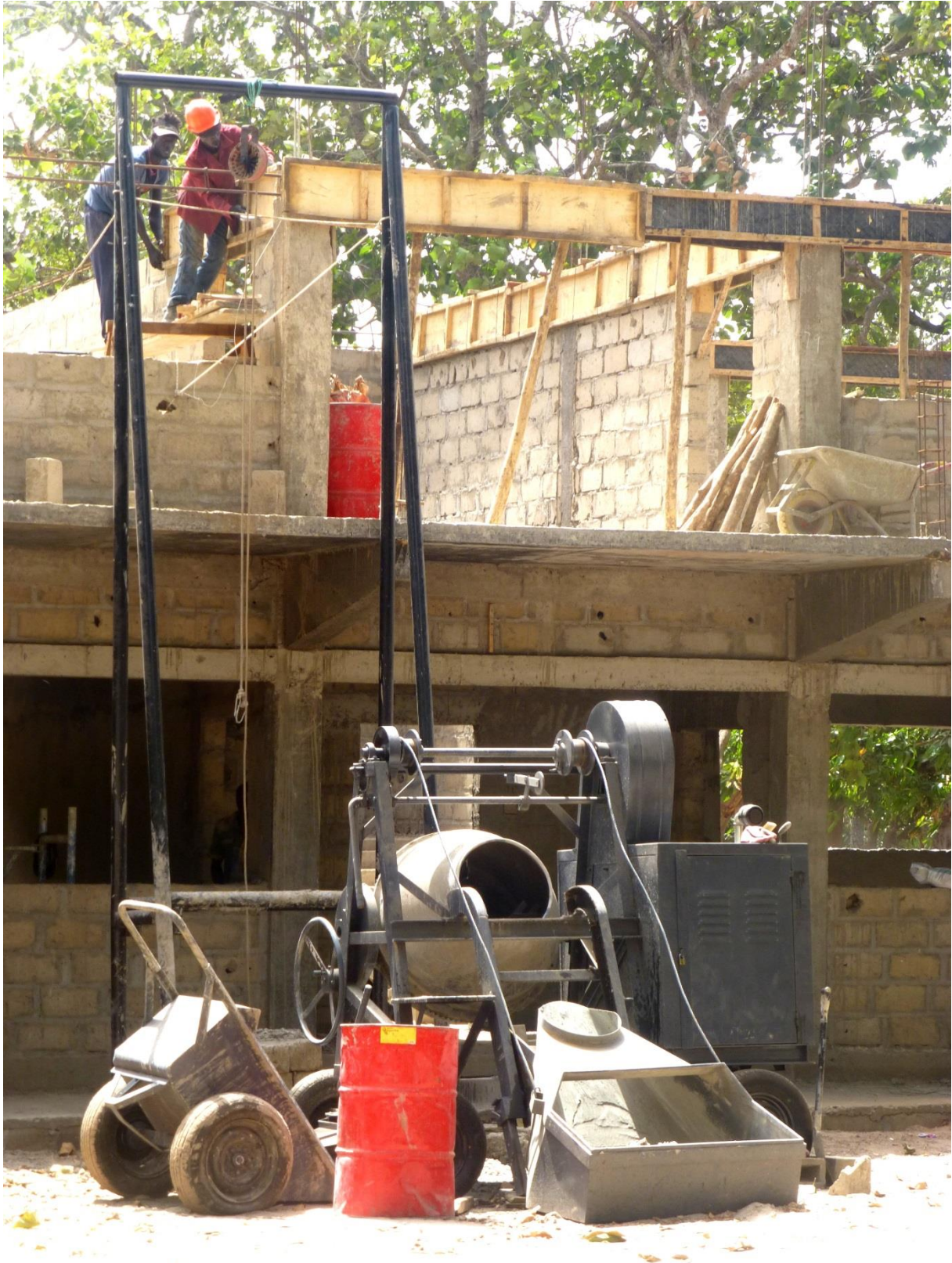
We provided a loan to three small contractors for buying more professional machinery.
